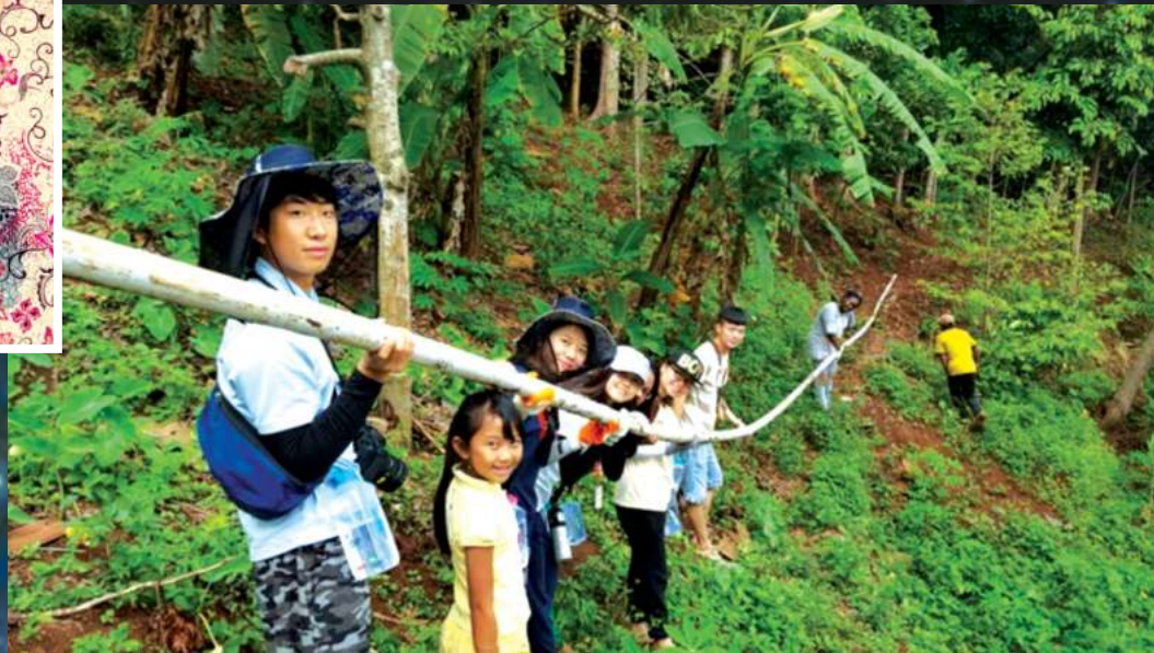
Helping local villagers fix their water supply system 協助當地村落解決供水系統問題
